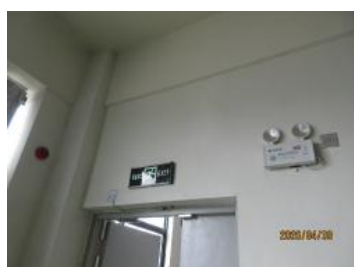
Emergency Light, Exit Sign and Fire Alarm.JPG
