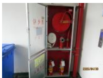
Fire Hydrant and Fire Extinguishers.JPG
