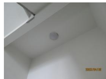
Emergency Light in the Staircase.JPG
