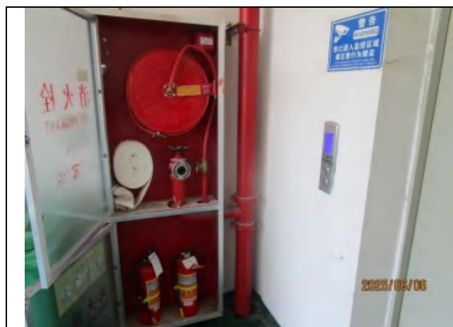
Fire extinguishers and fire hydrant
