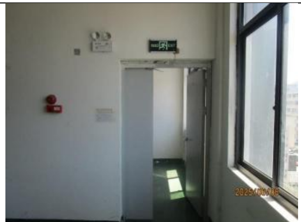
Evacuation exit with exit sign and light
