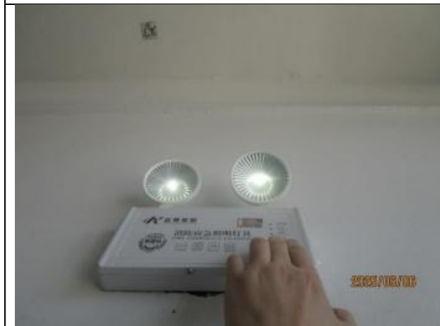
Emergency light testing
