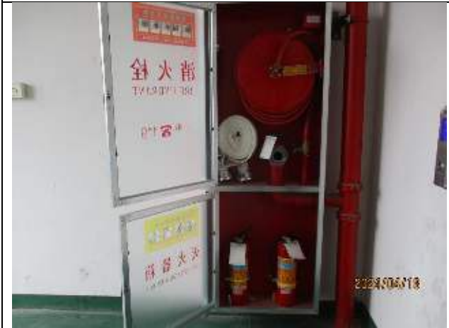
Fire extinguishers and fire hydrant
