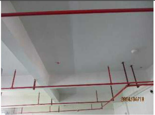
Fire sprinkler and smoke detector
