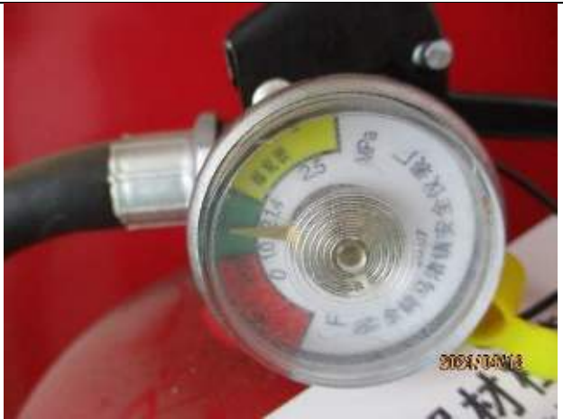
Fire extinguisher pressure was OK
