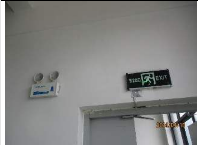
Emergency light and exit sign
