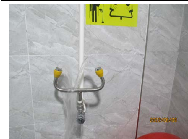
Eye washing station
