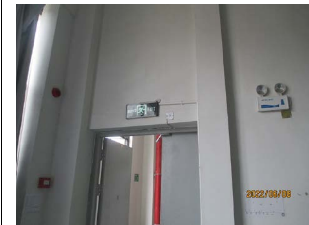
Exit sign and emergency light and fire alarm
