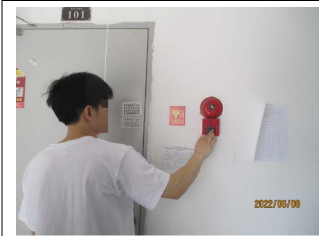
Testing fire alarm
