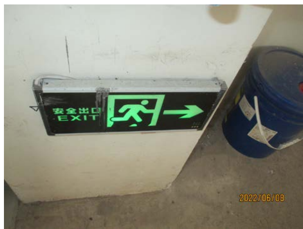
Evacuation indicating sign
