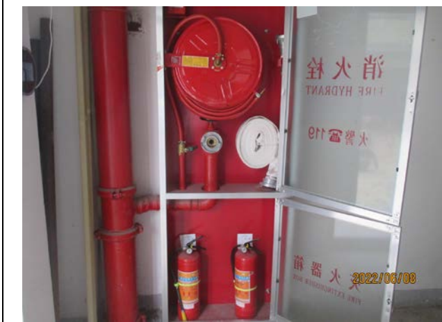
Fire hydrant and fire extinguisher
